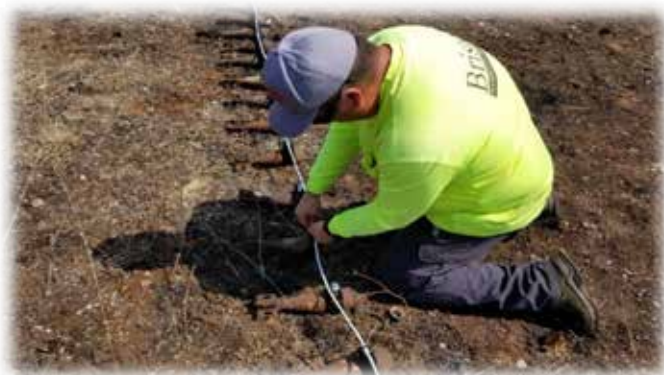
BBNC Shareholder Corey Lind prepares charges on unexploded ordnance (UXO) items for explosive demolition at Joint Base Lewis-McChord.
