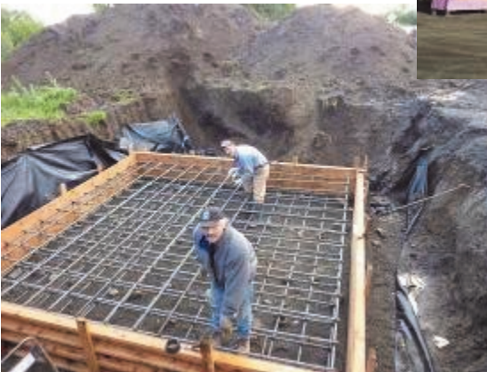
John Bennett, Jr. and William Tennyson, Jr. get ready to pour concrete for the foundation of the wind turbine.
